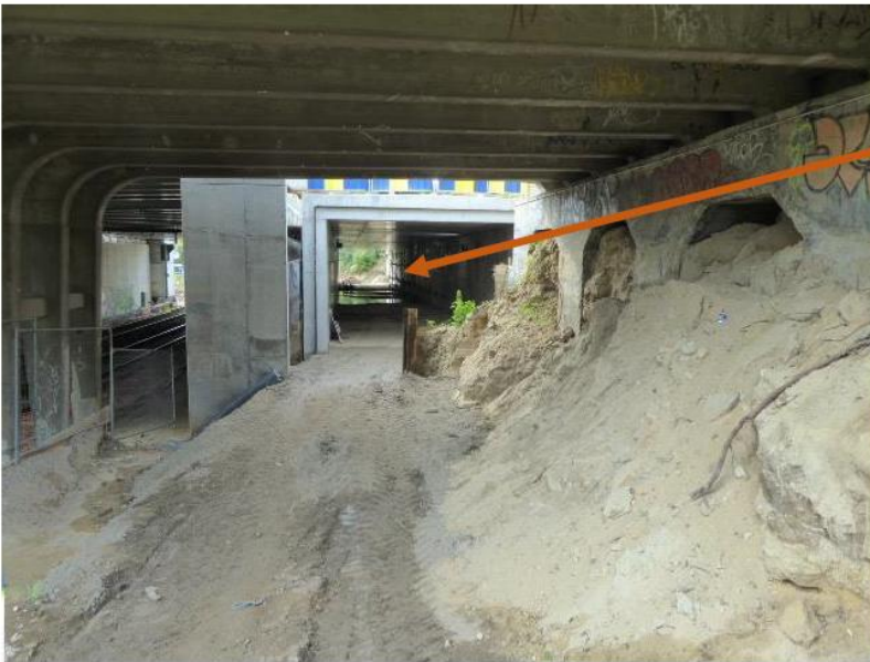
Tunnel ICR & ICC Future exploitation
